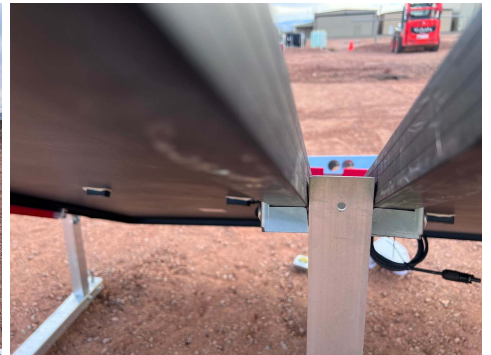
PHOTO 12: Middle brackets after testing
