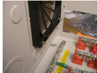
E-Panel earth ground bus (AC & DC)
