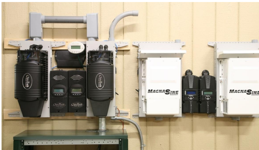
OutBack and Magnum horizontal stacked systems
