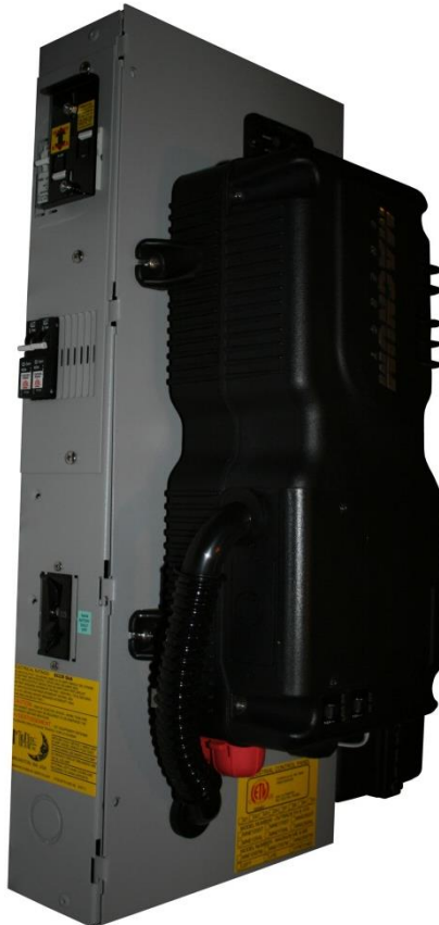
E-PANEL FOR MAGNUM MM SERIES AS INSTALLED
