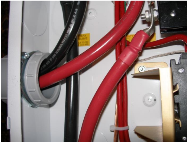
Wire exit to inverter
