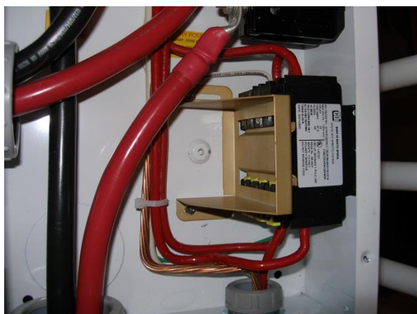
Din Rail mounted breakers
