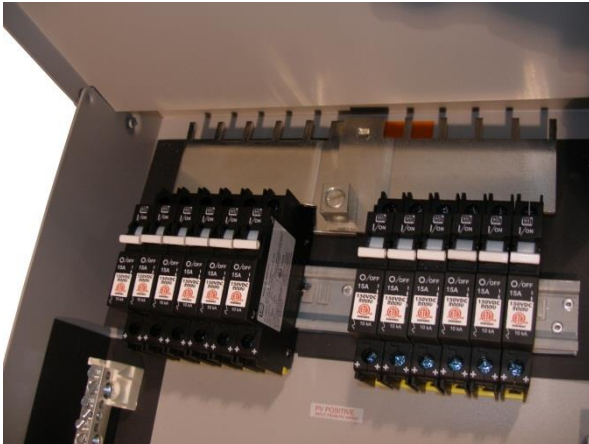
MNPV12 with breakers combined
